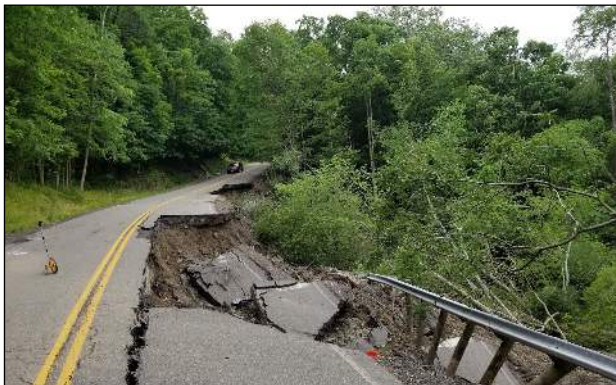
County Road 26 Slip—Spring 2023
