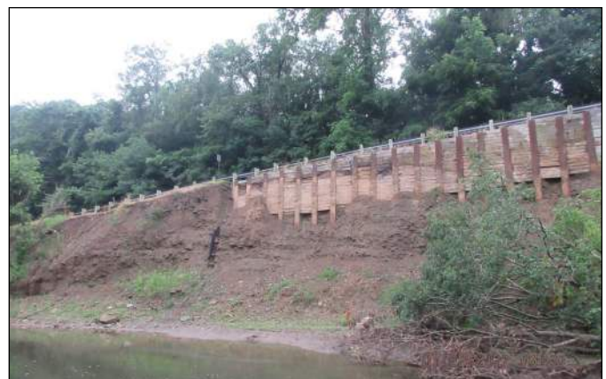
County Road 74 Slip—Existing Driven Pile Wall Exposed by Severe Erosion
