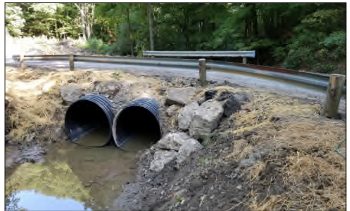
TR 61 — Dual 5' HDPE Pipes
